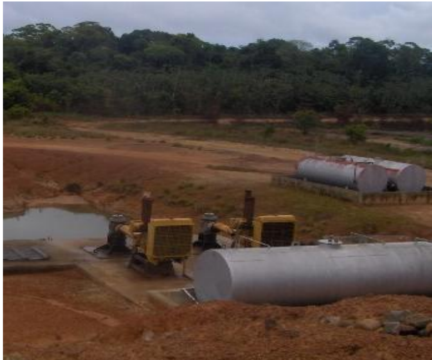
Plate 8.3 Fuel Tanks in Containment Structure at Haney Farm
