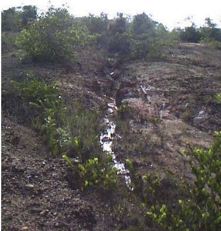
Plate 9. Deep erosion channels draining into seasonal streams along southern slope. Note sparse vegetation.
